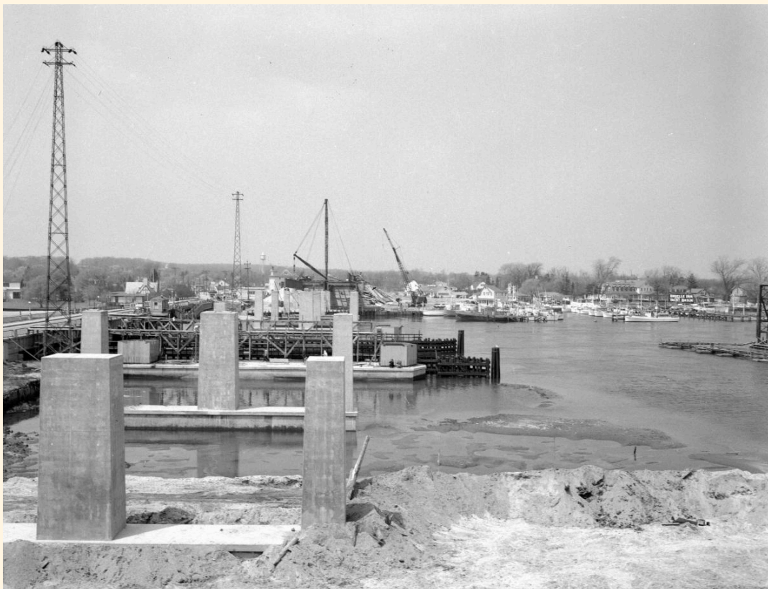
(above) New Highway 35 Bridge Foundations being constructed as viewed from the Point Pleasant side of the river.
