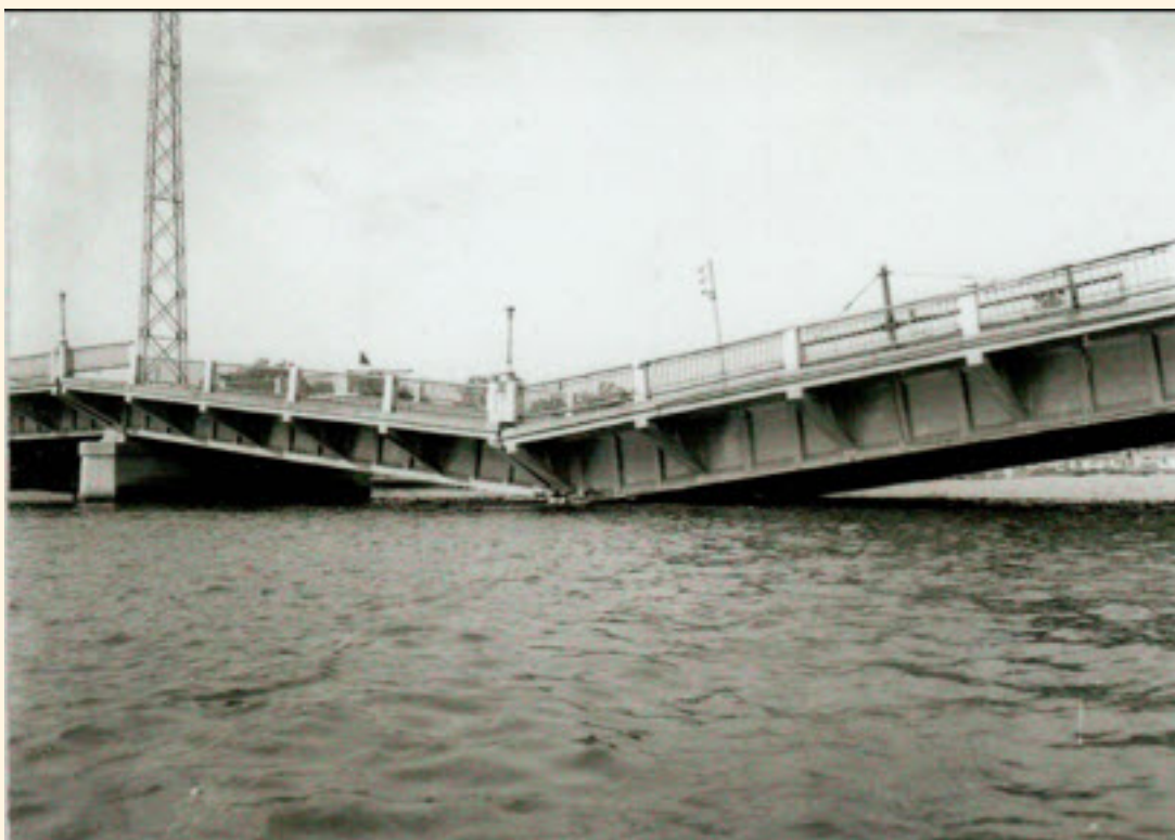
(above) Span failure of the Highway 35 bridge in 1946
